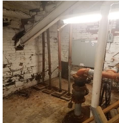
Pump Room Under Stairs
