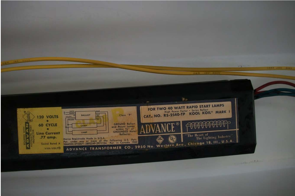
PCB light Ballast
